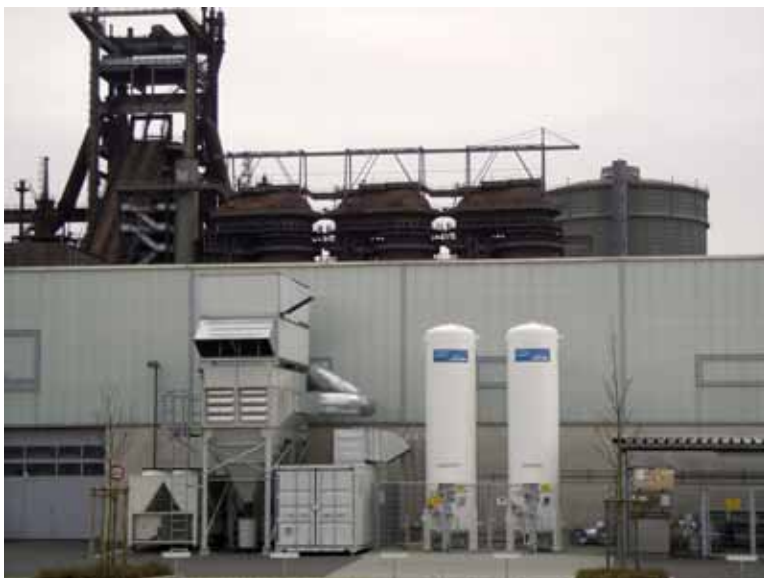
The GS40 is installed outside the factory providing more space, less noise and a cleaner working environment.
