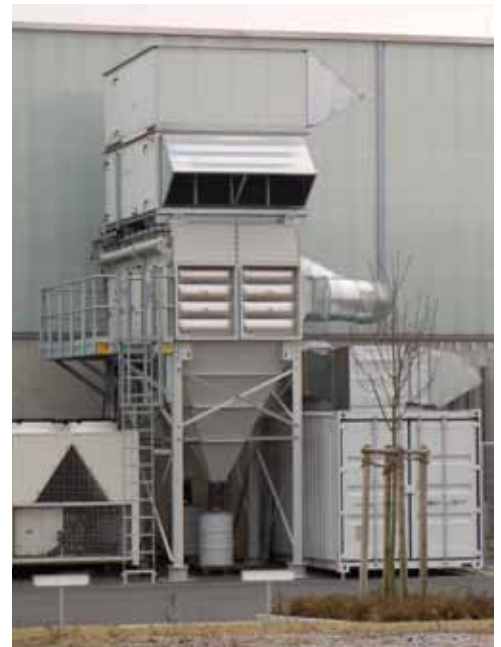
A Farr Gold Series® GS40 dust extractor located at Thermico's factory, in Dortmund, Germany. The most sustainable dust collector from Camfil APC on thermal spray.
