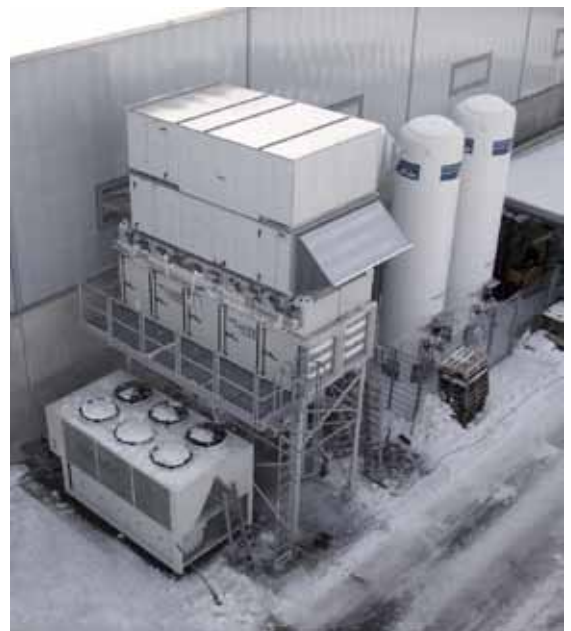
A view of the heat exchange system installed above the dust extractor.
